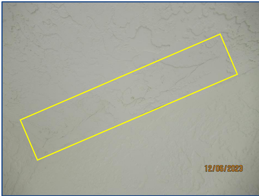
Photograph No. 18: View of cracks in the exterior ceiling finishes observed in the balcony of Unit 408.
