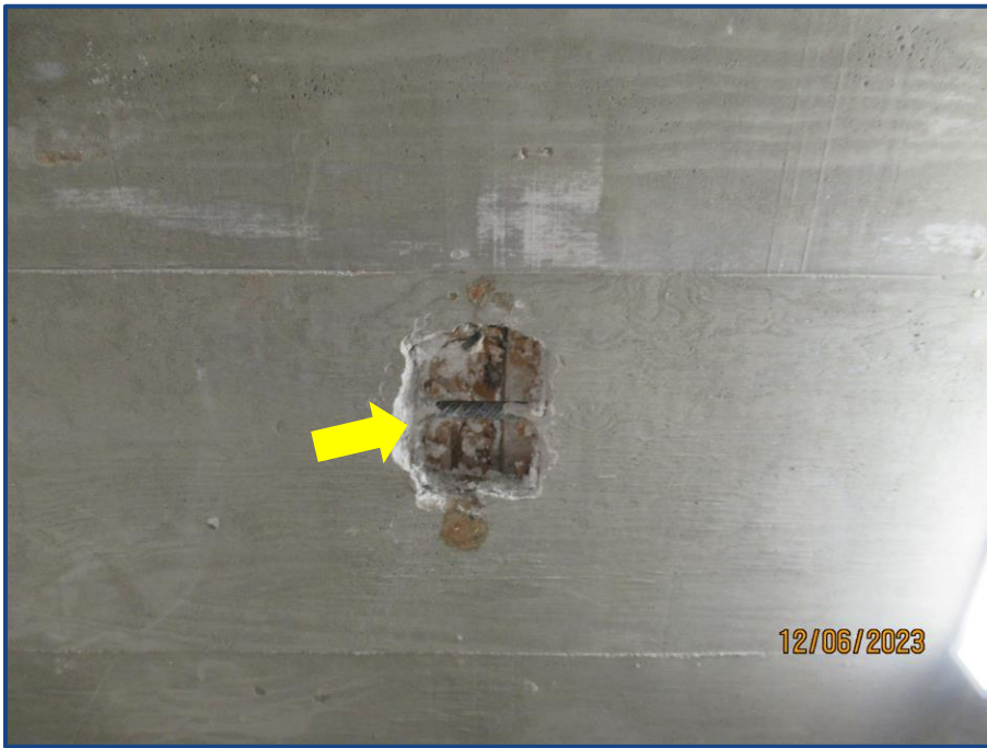
Photograph No. 14: View of exposed steel reinforcement in the ceiling slab located in the electrical room.
