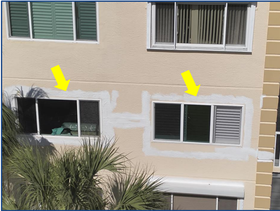
Photograph No. 10: View of previous patch repairs.
