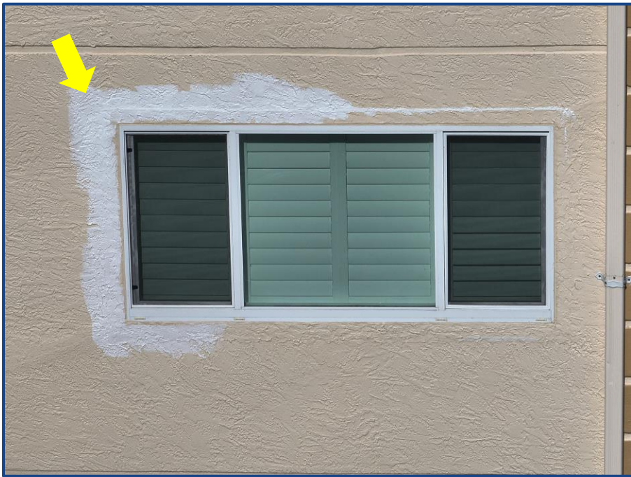
Photograph No. 12: View of previous patch repair.
