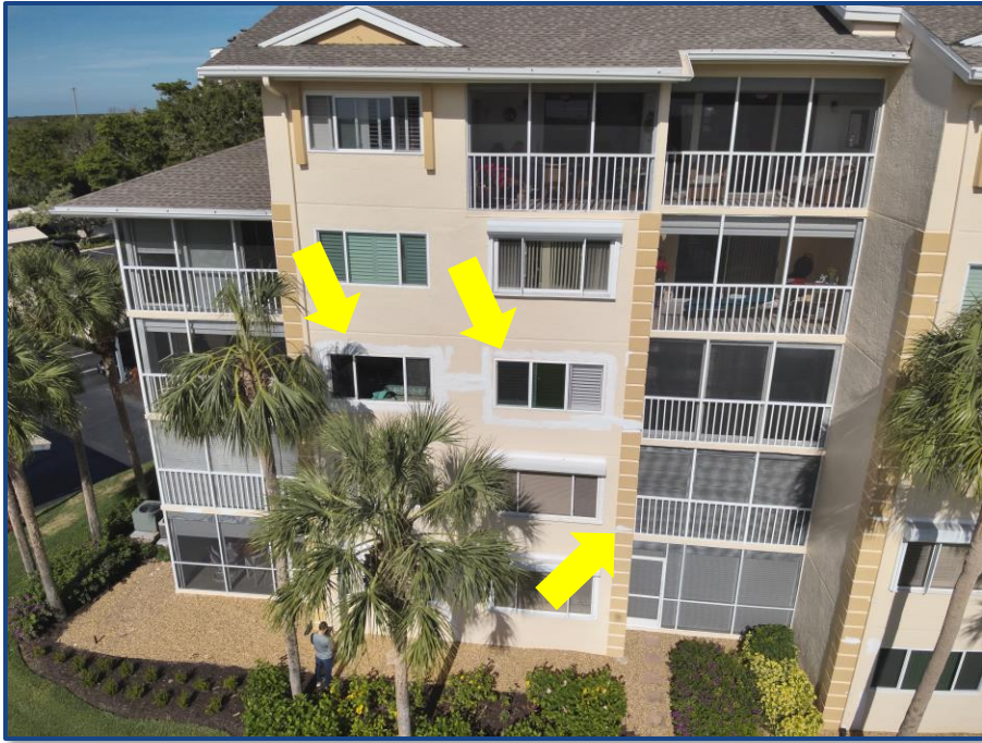
Photograph No. 9: View of previous patch repairs.
