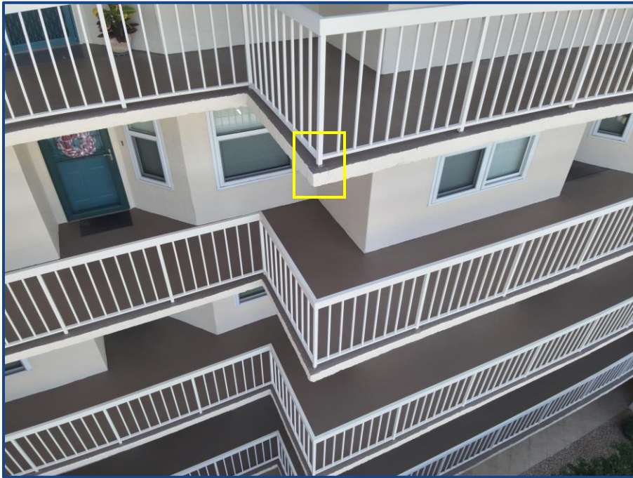
Photograph No. 8: General view of the exterior walkways and cracks/spalling in the exterior walkway corner on the fifth floor.
