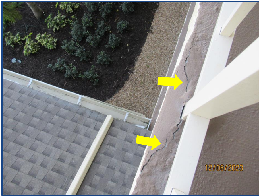
Photograph No. 27: View of cracks/spalling along the exterior walkway edge on the fourth floor.
