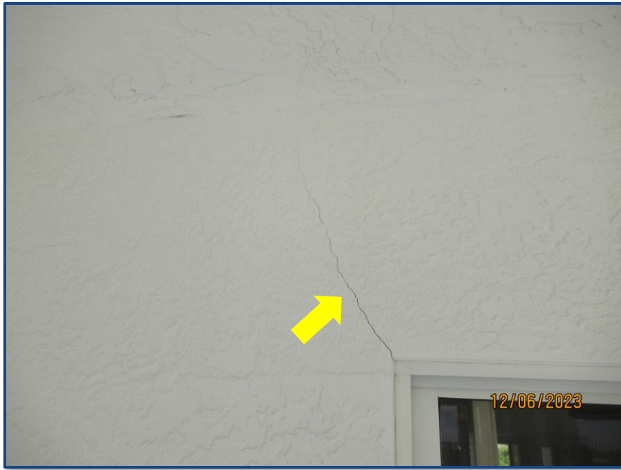
Photograph No. 17: View of crack in the exterior stucco wall finishes observed in the balcony of Unit 408.
