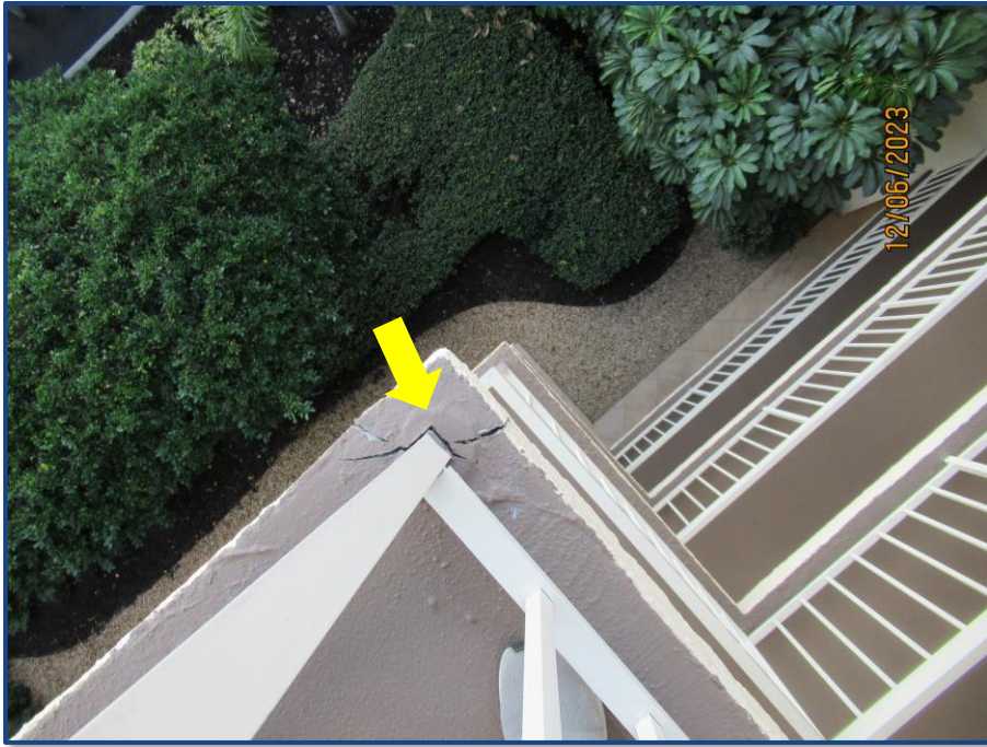
Photograph No. 25: View of cracks/spalling in the exterior walkway corner on the fifth floor.
