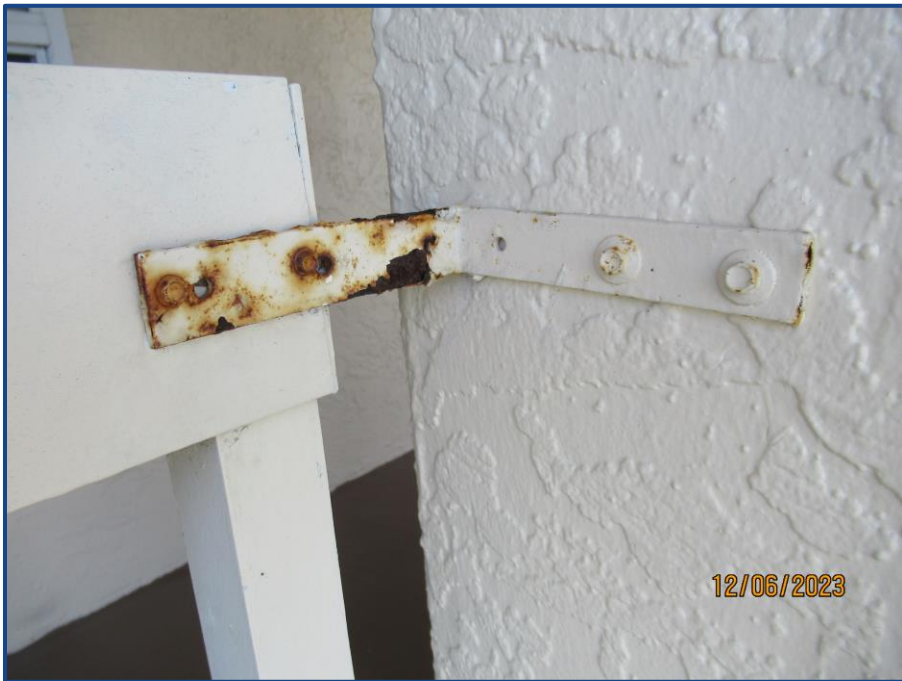
Photograph No. 24: View of corroded steel bracket observed on the 5th floor near the western end.
